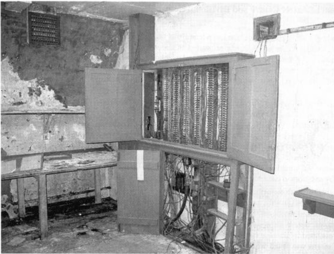
Brighton; Switchboard room
